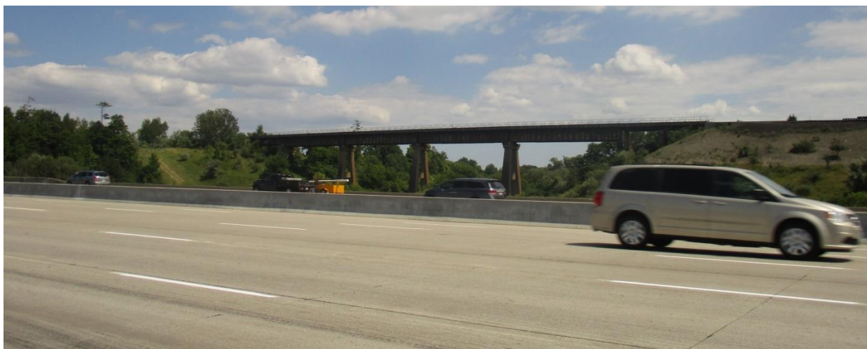
Figure 14: York CNR Bridge Looking South, Near Islington Avenue, a 1962 Rail Bridge Over the Humber River.
