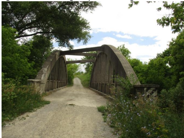
Figure 12: Wiley Concrete Bowstring Arch Bridge over the Humber River at Claireville Conservation Area.
